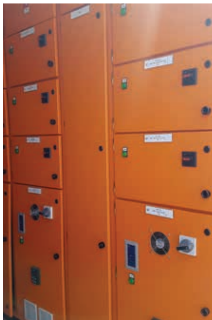
Part of WEG Automation's SC 300 MCC rack.
