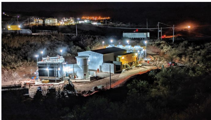
A modular approach was adopted for the surface air cooling systems to provide flexibility to accommodate the surface geography, save costs and minimise site construction time.
