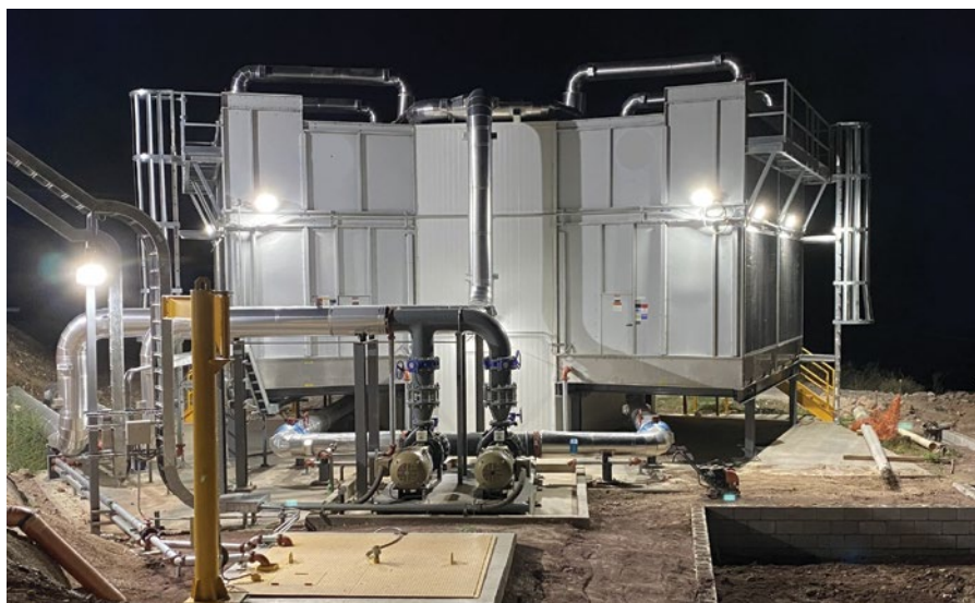
Given the constraints of the surface geography, both surface air cooling systems and surface fan stations had to be compact.
