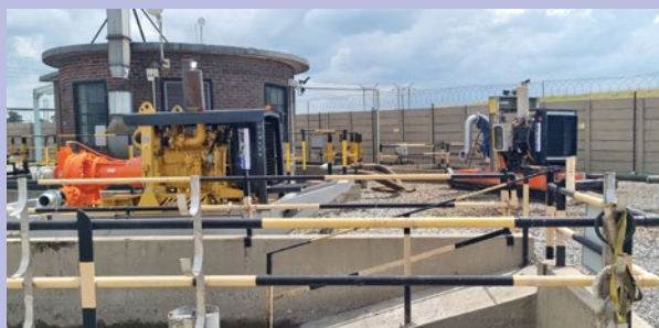
Integrated Pump Rental selected, delivered, commissioned and had two Allight Sykes dewatering pump sets to provide bypass water lines at the customer's pump station.
