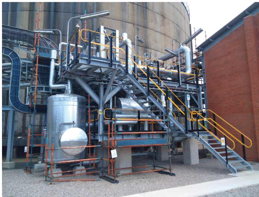
The new Rail-Loading Condenser system lowers operational costs, minimises flaring and ensures statutory inspections can be carried out safely.
