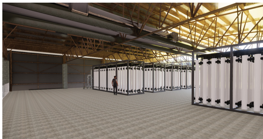
A view of the ultrafiltration plant that removes any particles, pollutants and pathogens/germs smaller than 10 µm.
