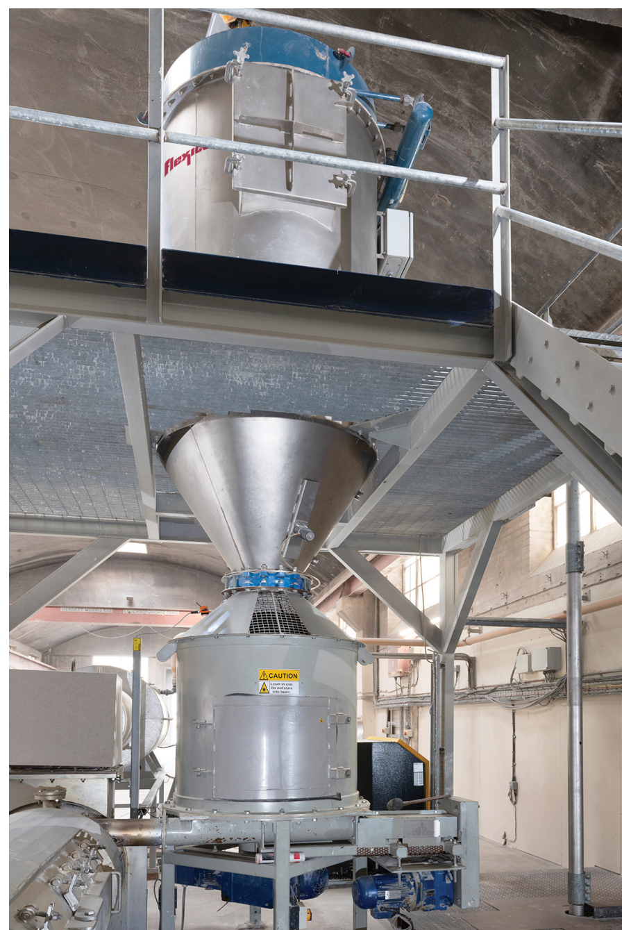
A 30 m conveying line transfers wet, abrasive mica powder from the wet process on the floor below into the filter receiver, which separates the material from the conveying air.
