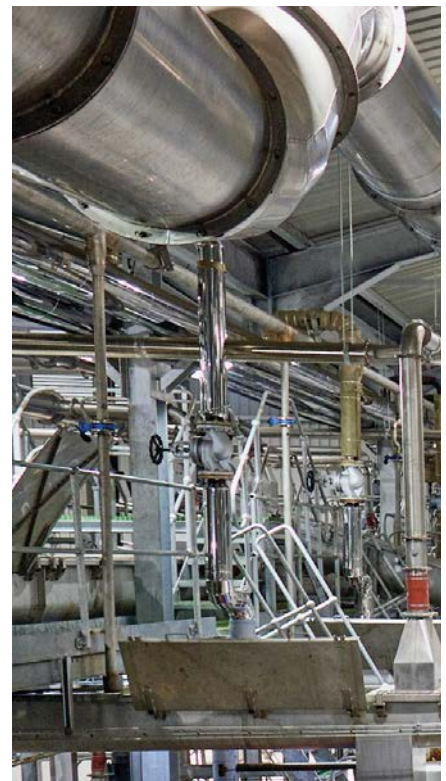
A steam plant for the food processing industry with multiple offtakes.
