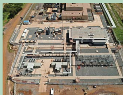
Hitachi Energy has delivered a state-of-the-art power electronic converter that stabilises the mine's connection to the grid.
