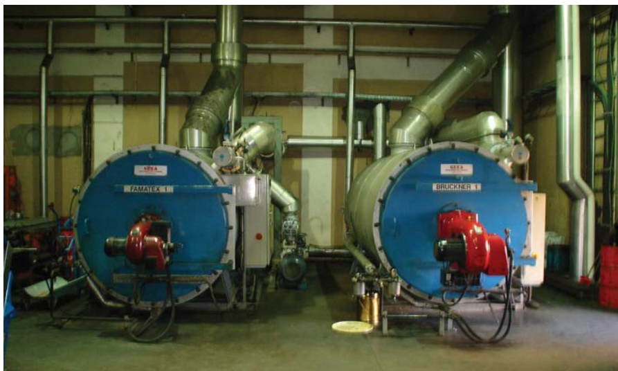
A thermal oil heater plant that uses liquid fuel burners to heat and circulate high-temperature oil through equipment such as textile machinery.
