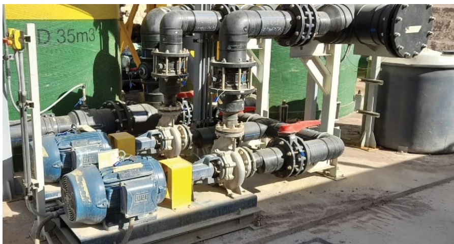
SAER NCB super-duplex end-suction pumps installed in a desalination plant.
