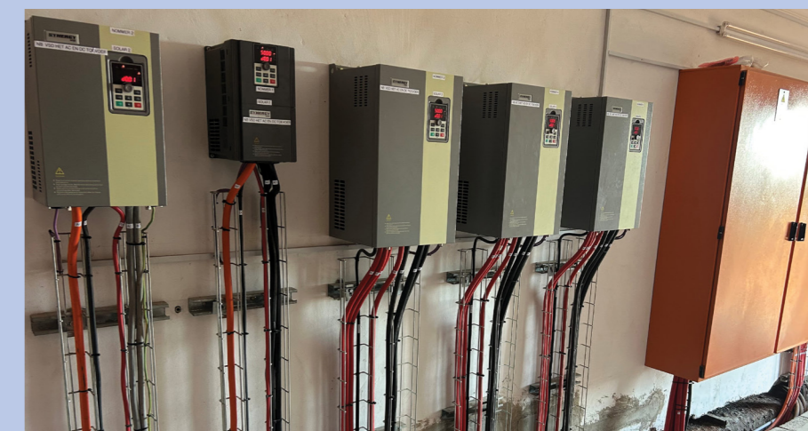
BMG and Agrico have collaborated to improve compatibility between BMG Synergy PI500 variable-speed drives (VSDs) and Agrico's Web Control platform.
