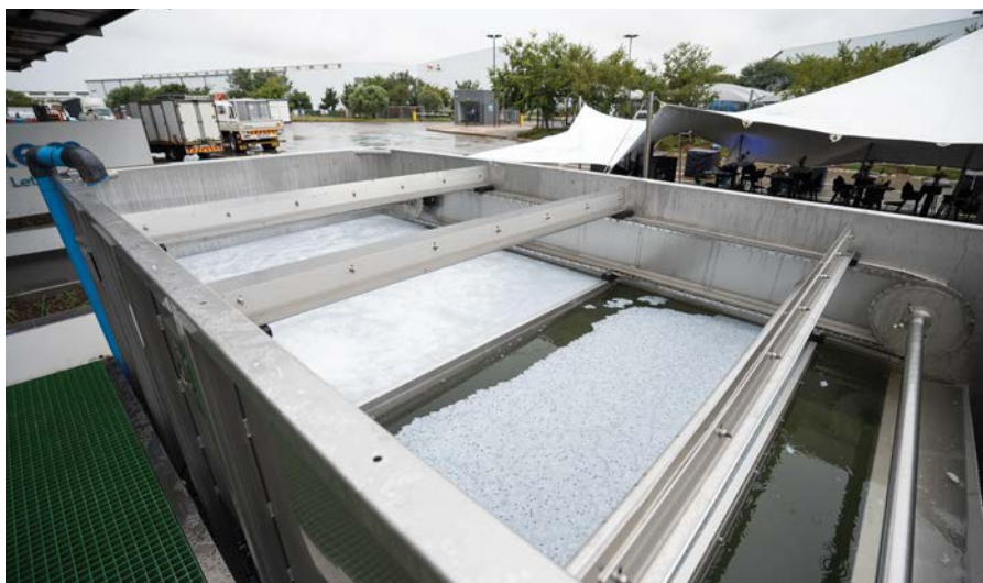
DAF water treatment efficiently removes total suspended solids (TSS); fats, oils, and greases (FOG); and particulate-associated biochemical oxygen demand (BOD) from wastewater streams.
