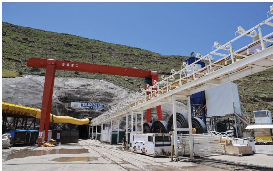
Hard-rock tunnel boring was used to create the 5 m diameter Polihali Transfer Tunnel.
