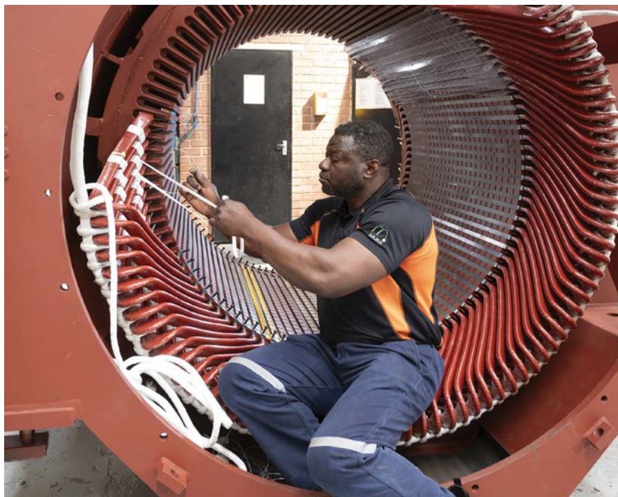
Marthinus & Coutts (M&C) is completing alternator overhauls and stator-winding rehabilitation on 17 identical alternators for gas-powered energy generation.
