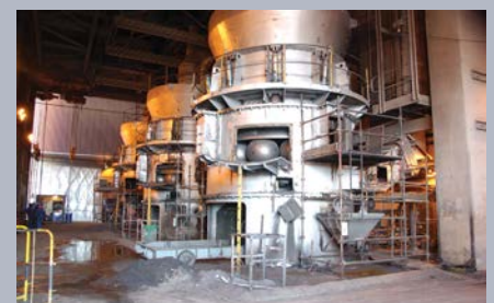
Experience at Babcock demonstrates that engineering-led rehabilitation programmes can restore milling plant stability without significant capital investment.
