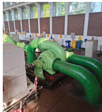
The Jericho Pump Station in Mpumalanga, built in South Africa in 1967 and still in operation, reliably delivers water to communities and industry.
