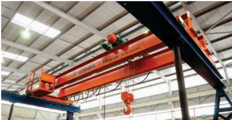
Typical Condra double-girder overhead crane under test.
