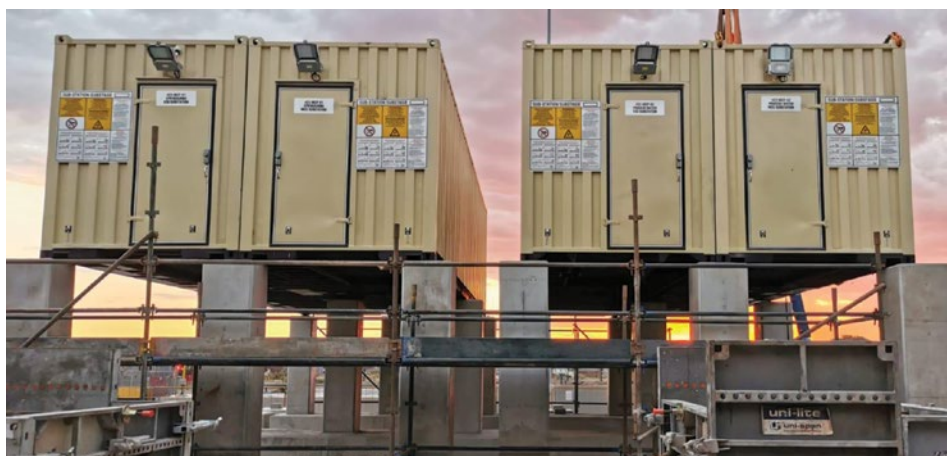
Containerised Motor Control Centres form part of Zest WEG's scope of supply.
