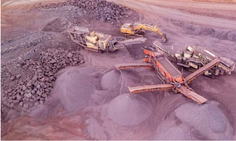
Afrimat is busy with mobile crushing at its facility in the Northern Cape.
