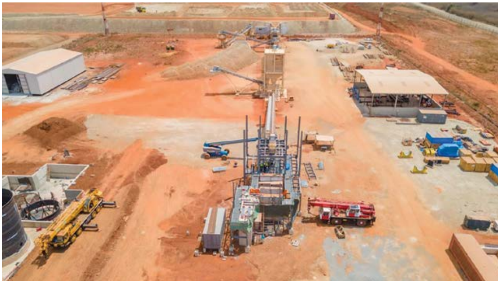
NCP-manufactured grinding circuit installation at Singida.
