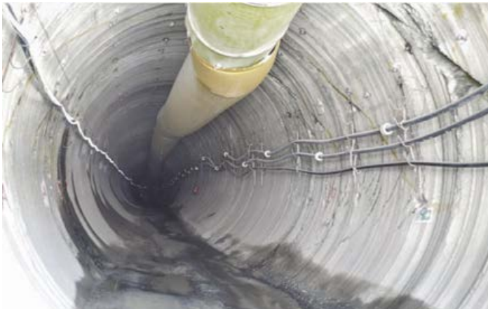
Above: TBM decline in NRHR. Exploration project using drilling and blasting and MTB methods, J Walls, SANGOT 2022.
