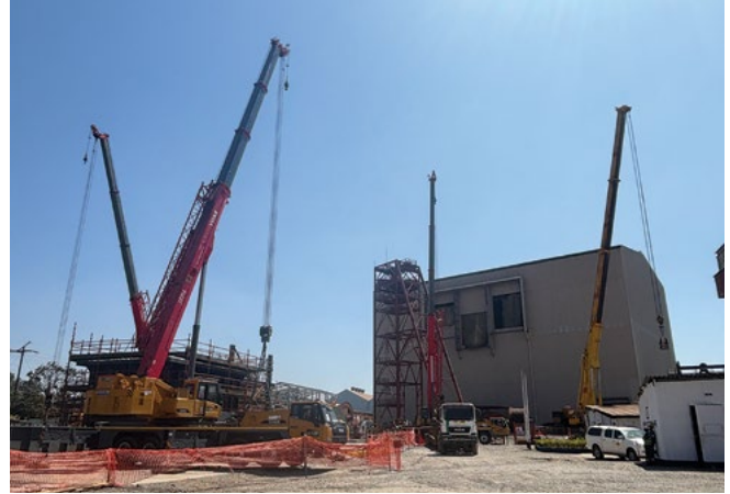
With the new winder house visible in the background, four mobile cranes lift steel sections for the pre-assembly of the headgear.
