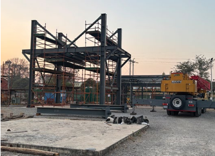
Structural steel components of the ore loading bin prepared for assembly on site.
