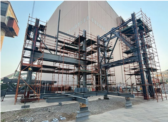
Pre-assembly of the headgear centre column is underway, ensuring alignment and structural integrity before installation.
