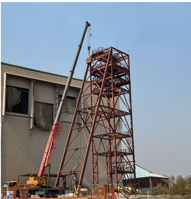
An 80 ton mobile crane lifts a section of the ore loading bin as part of ongoing structural installation activities.
