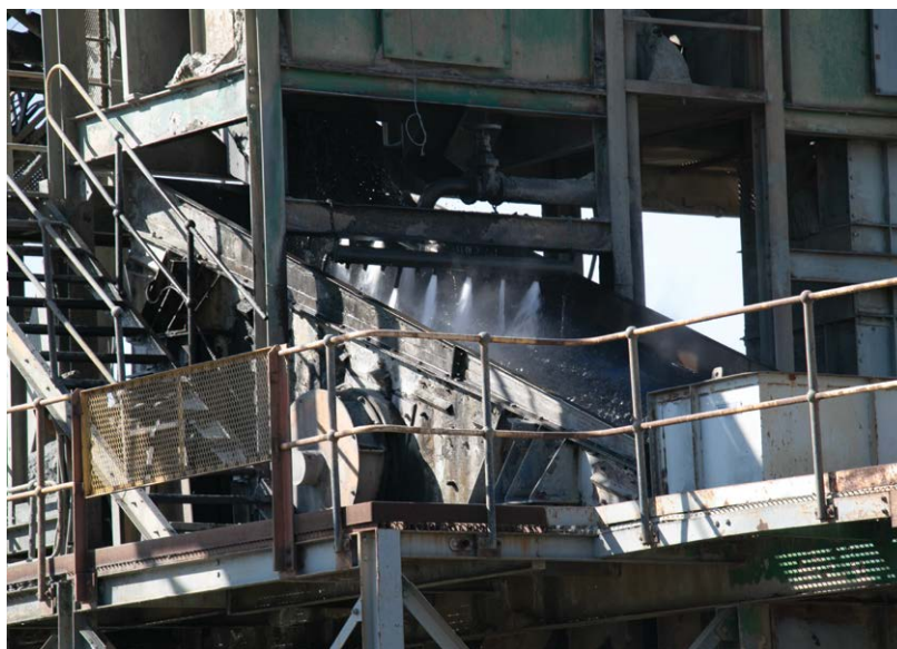
In order to produce the various products for the road building industry, a washing process is needed to meet the requirements and specifications of the saleable products
