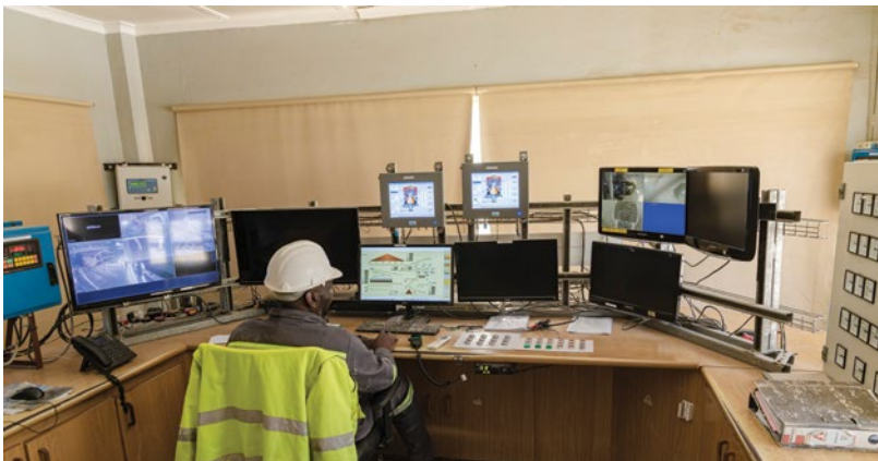
Peninsula Quarry continuously monitors plant performance, throughput and equipment efficiency to support reliable, data-driven production management.
